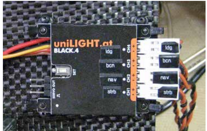
Controller installed on equipment tray. Identification tags placed on unit and attaching plugs for easy reference.
